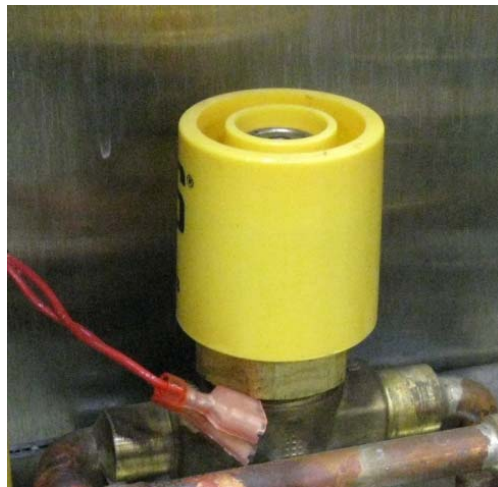
Figure 4-27: Coil Magnet on Solenoid Valve
