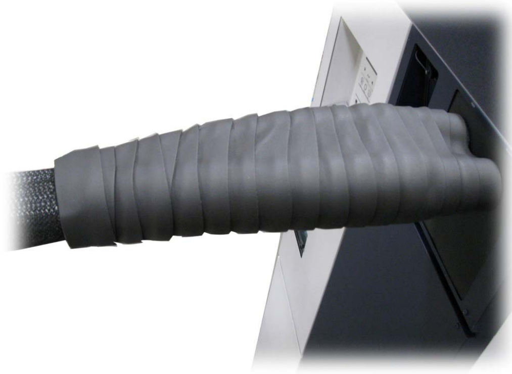
Figure 4-36: View of Armaflex Insulating Tape on Refrigerant Line Bundle on Polycold Cryochiller
